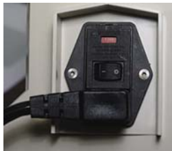
Power on the Generator.
